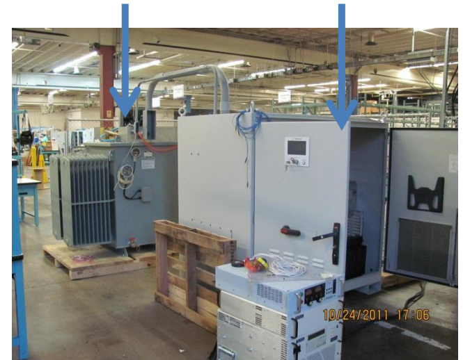
HV Enclosure LV Enclosure
