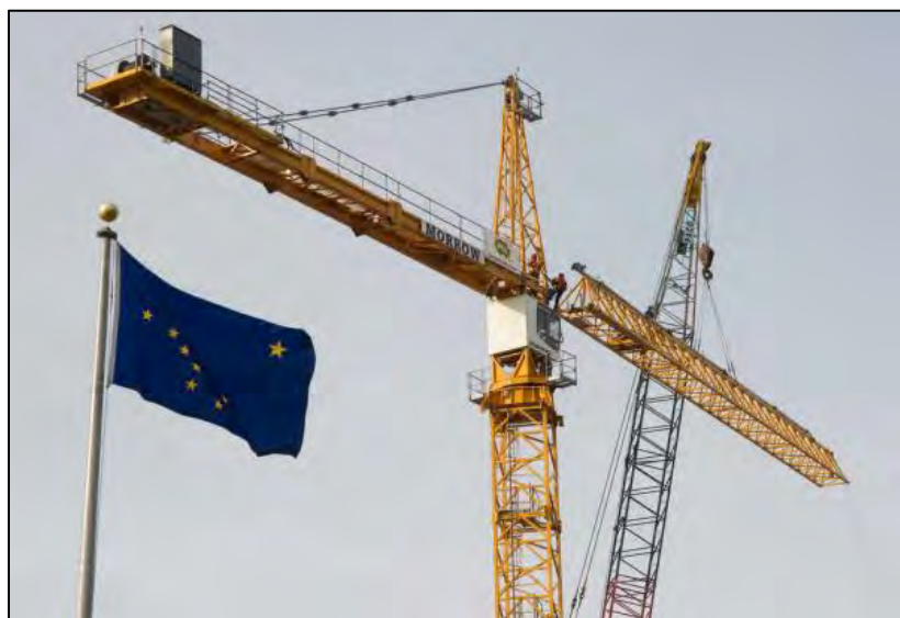
The State Library, Archives and Museum project's crane dominates the Juneau skyline these days. Photo: Juneau Empire
