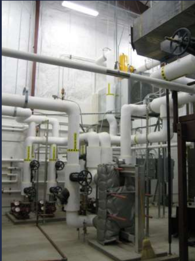
Biomass heat system
